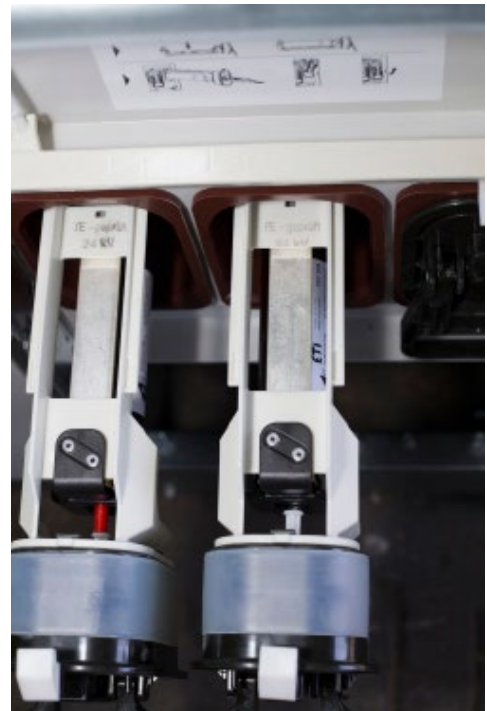
Connection in indoor switchgear, example:
